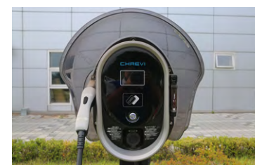
Electric Vehicle Charging Station
